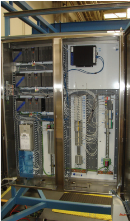
Control Cabinet with JumboSwitch 25 Chassis
